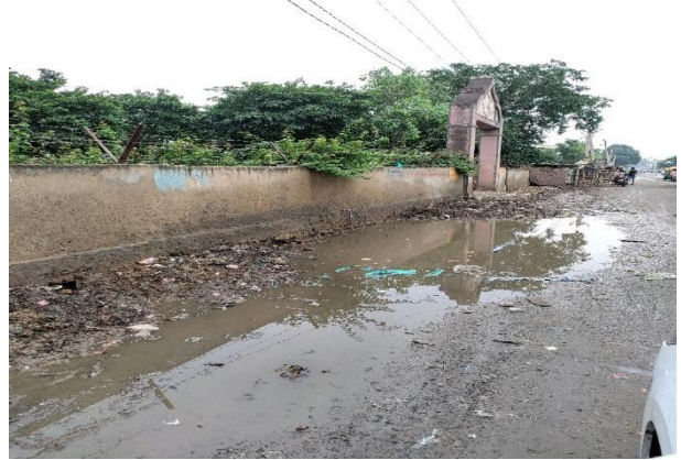
Figure 4.39 Sewage near Road due to Lack of Drainage
