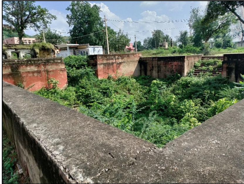
Figure 5.6 Baveri- Artificial Water Storages Structure (27°14'08.8"N 76°36'41.8"E)
